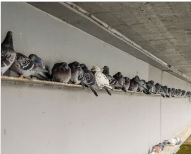
Figure 2: Pigeons colonising the undercroft of a bridge in high numbers.
